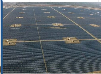
Quaid-e-Azam Solar Power Plant
