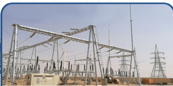
100MW Three Gorges Second & Third Wind Power Project
